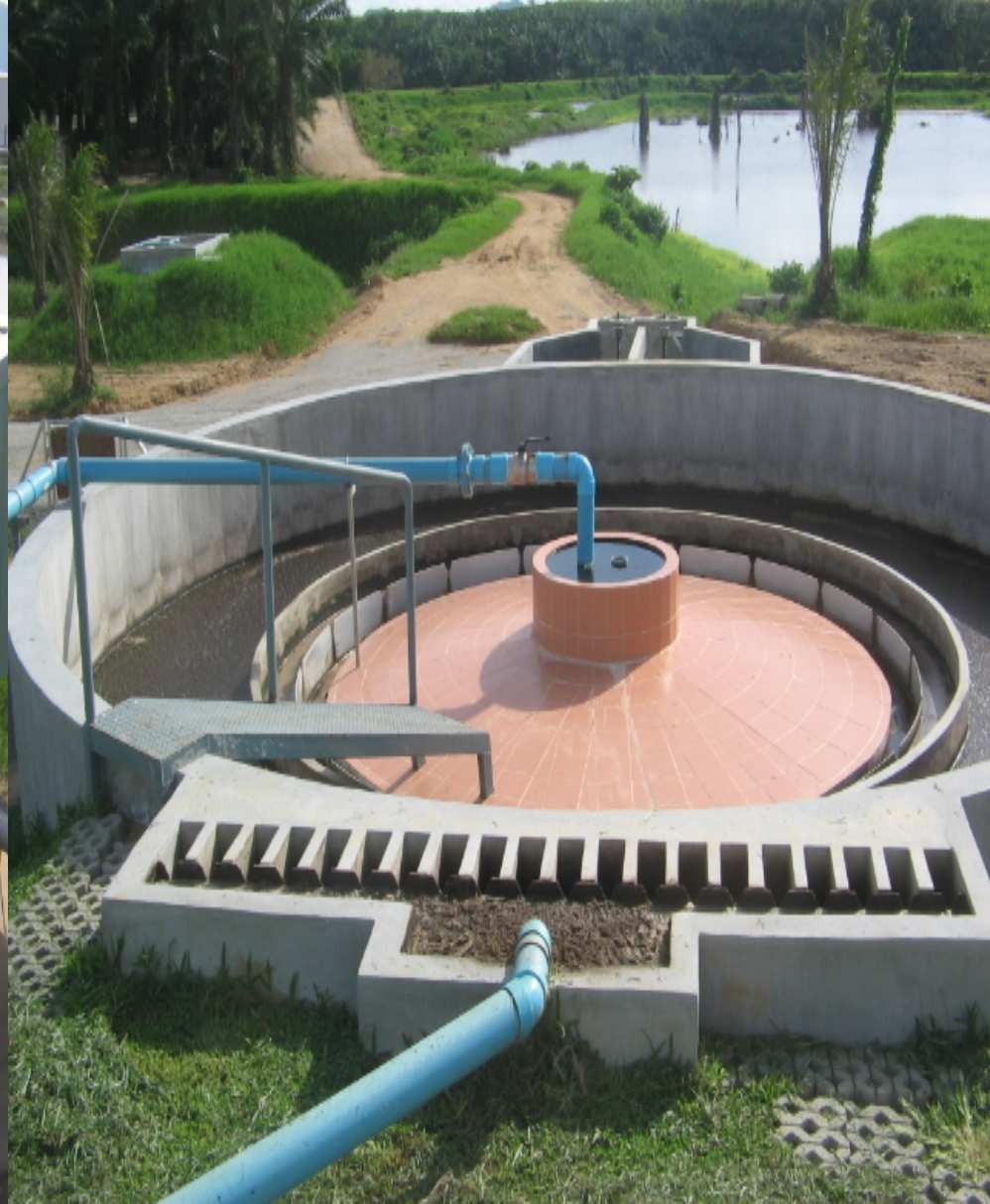
Appropriate + Up Flow Anaerobic Sludge Blanket, Thailand (A+UASBTh) Reactor
