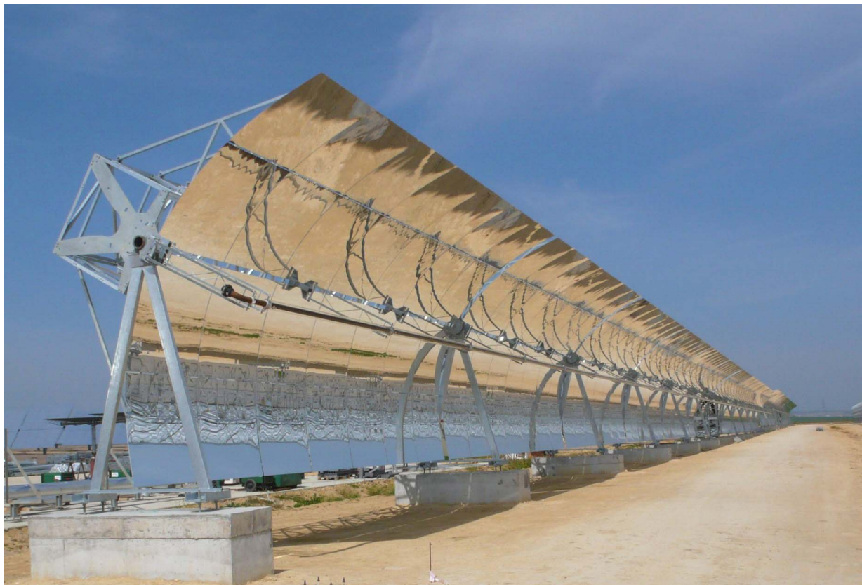
Cylindrical parabolic collectors (with the permission of Abengoa-Solucar)
