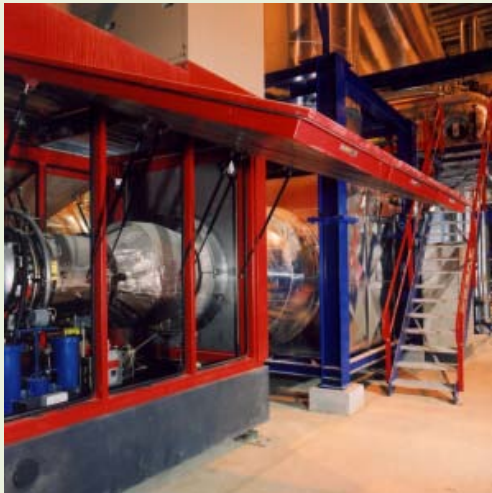
Figure 2 - Gas turbine and Recovery Boiler ( www.climaespaco.pt )
