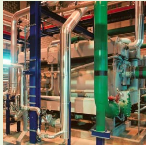
Figure 3 - Absorption chillers ( www.climaespaco.pt )
