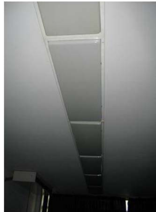
Existing Fixture-Acrylic Diffuser Type, T8, 2 x 36 W with Magnetic Ballast 150-250 lux
