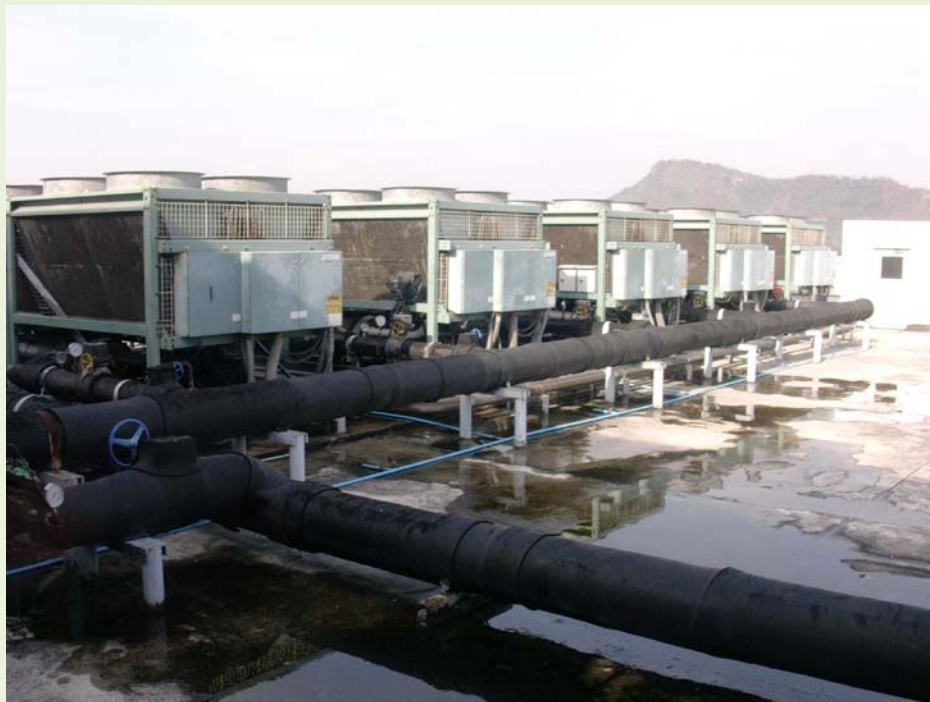
FIGURE B: PREVIOUS AIR-COOLED CHILLERS
