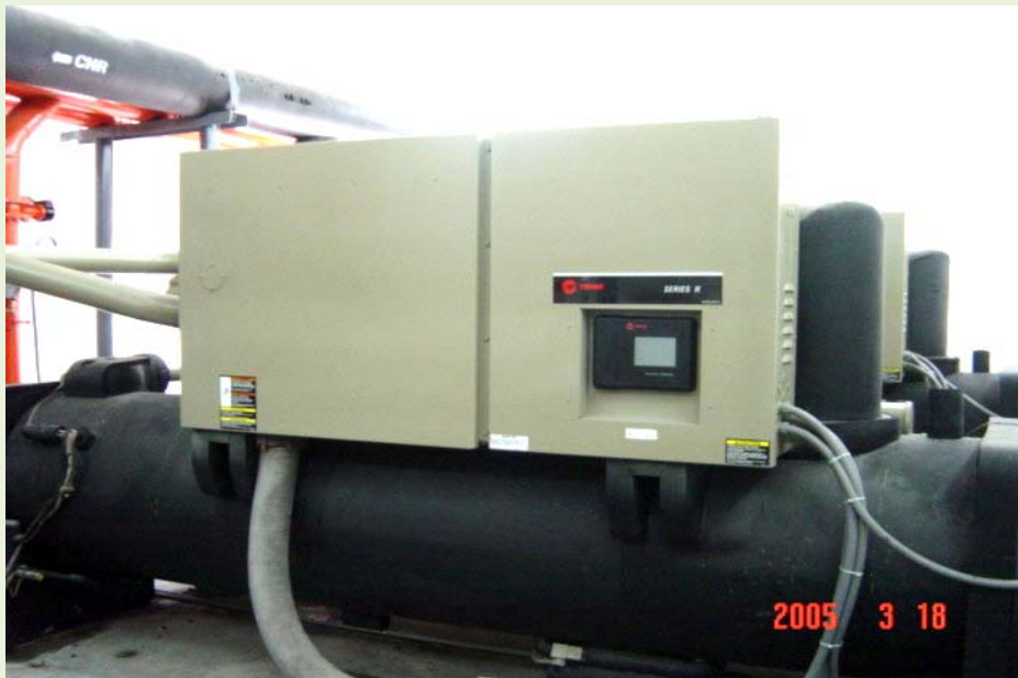
FIGURE D: NEW WATER-COOLED CHILLERS
