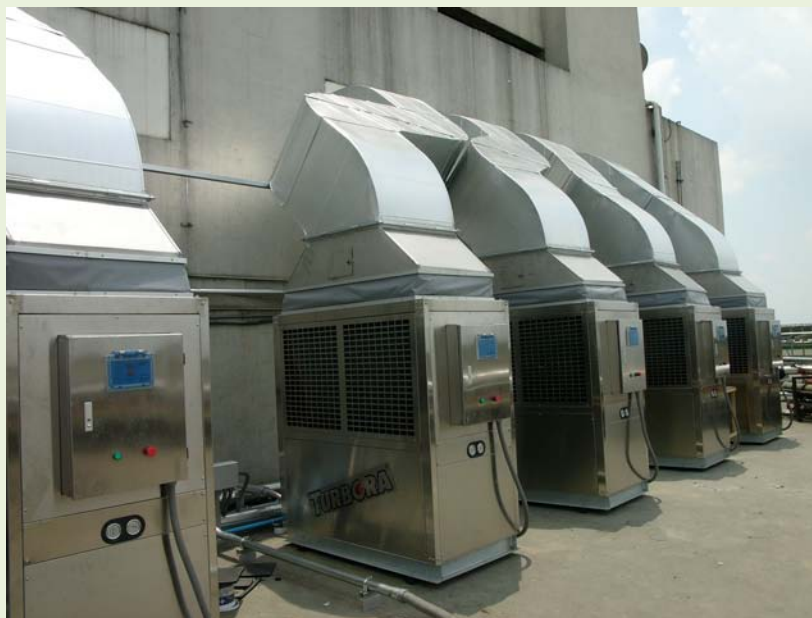
FIGURE C: HEAT PUMP ON THE ROOF TOP
